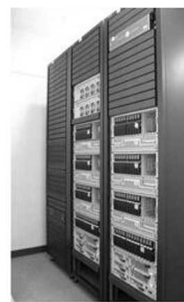
Fig 2 Developed low power consumption storage sub-system.
