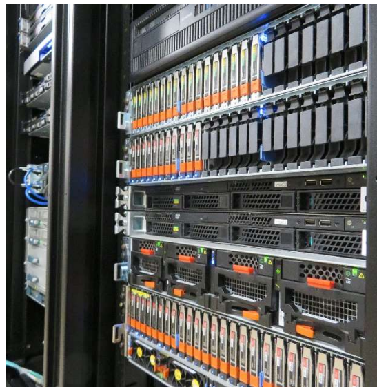
Figure RIEC server room
